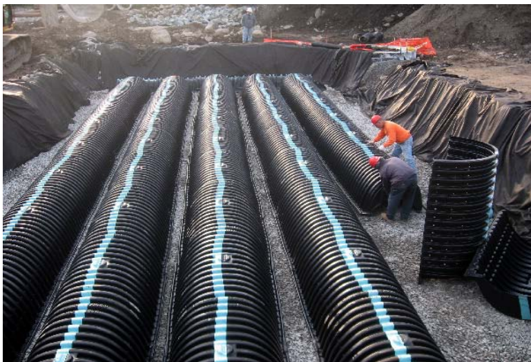
Figure 11-1: Subsurface Infiltration Systems
