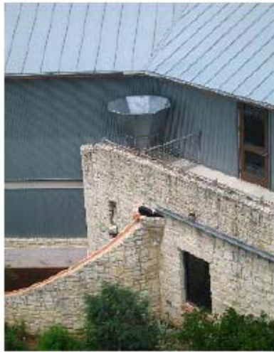
Downspout disconnection at Lady Bird Johnson Wildflower Center, Austin, TX.
